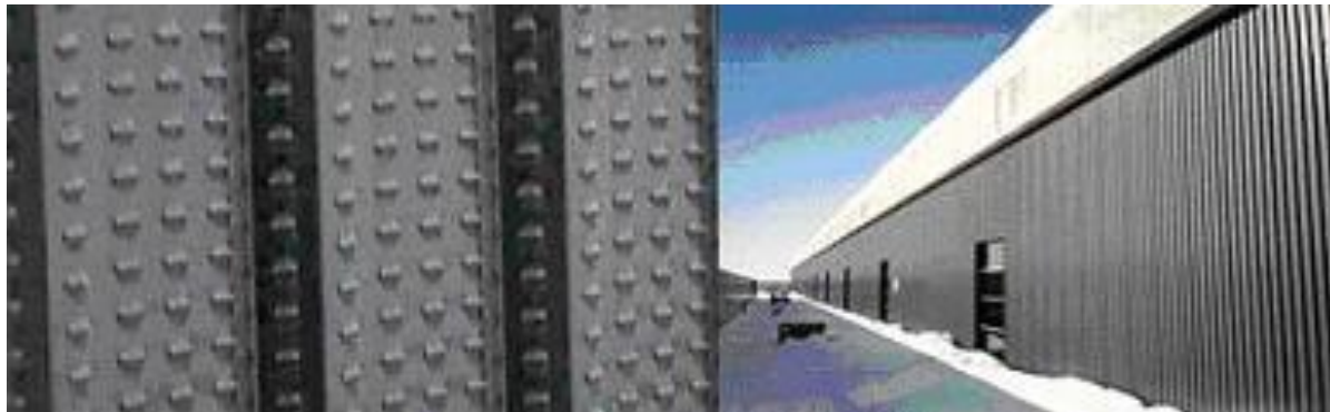
Hybrid energy using solar wall for lumber drying kilns
